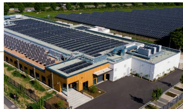
Data Center – LEW TelNet, Augsburg
